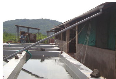
Fig. 1: Rain water harvesting through (U Shape) gutter
